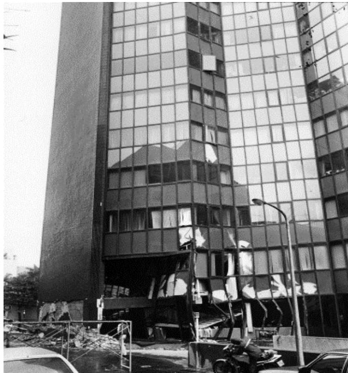
(b) Tilting and subsidence of a building when the seismic condition of the building changes moderately to a non-seismic condition (Hsu, 2019; Hsu, 2022b)
