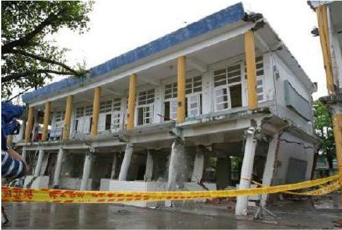
Figure 5. Imposed weak column-strong girder failure observed in the pushover test of a school building under seismic conditions (Hwang, 2009).
