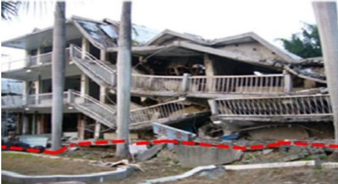
Figure 4. Collapse failure of the Guangfu Junior High School building in Nantou, Taiwan during the 921 Jiji earthquake (Hsu et al., 2023).
